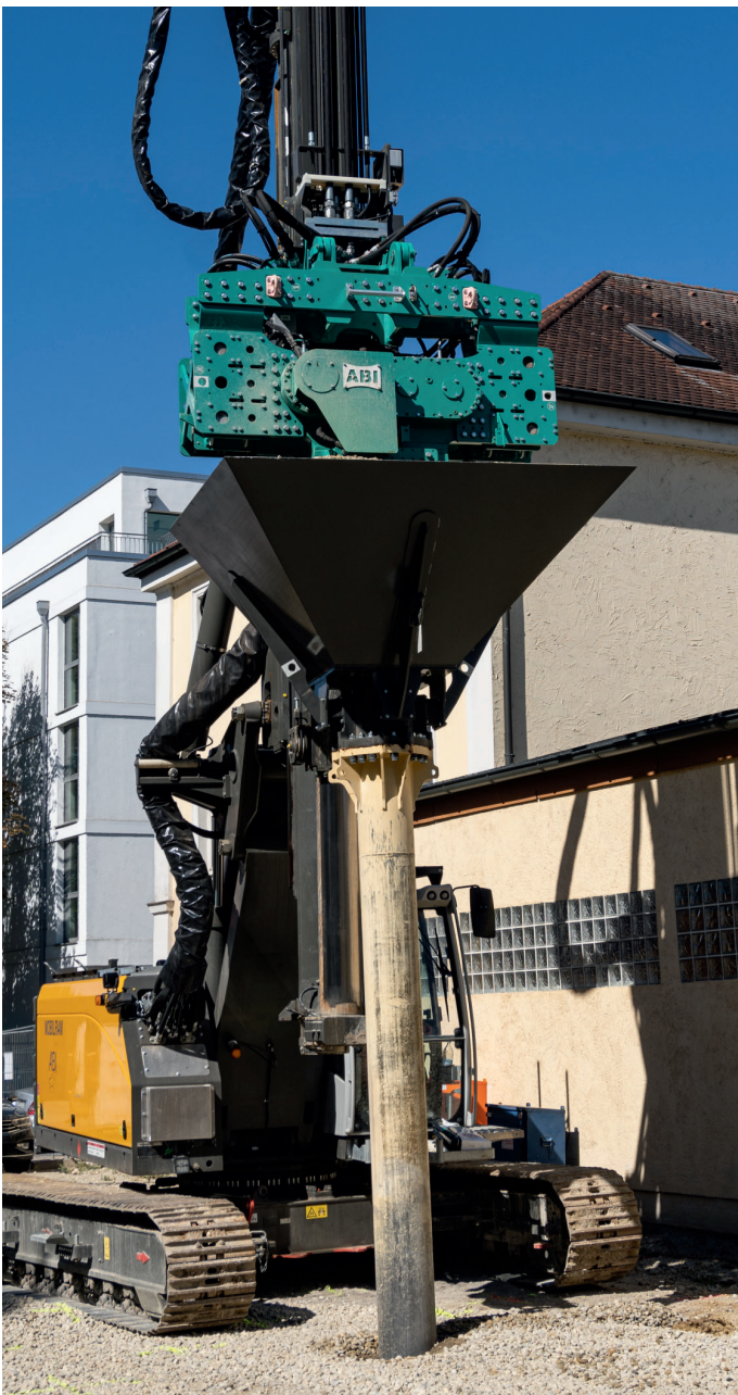
Photo: ABI MOBILRAM TM 13 with vibrator MRZV 15SD with hopper and probe installing stone columns
