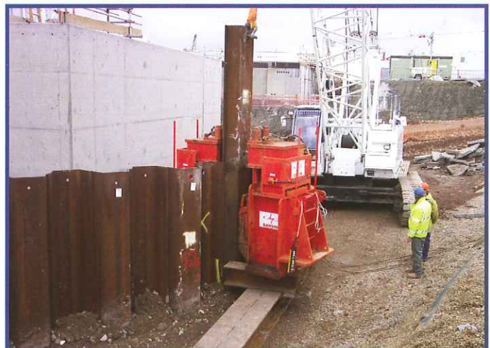
X400t Universal Pile Extractor pulling Arcelor PU25 sheet piles – Heathrow Airport Terminal 5, England
