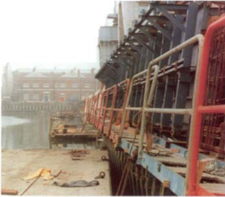
(above and front cover) 2 metre high pile cap over a total length of 1000 metres at the Royal Docks, Portsmouth. Main Contractor: Harbour and General Works Ltd. Client: Property Services Agency
