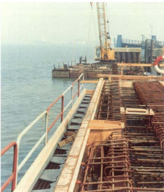
(below right and front cover) River wall on Thames near the tidal barrier at Greenwich. Main Contractor: John Shelbourne Ltd.
