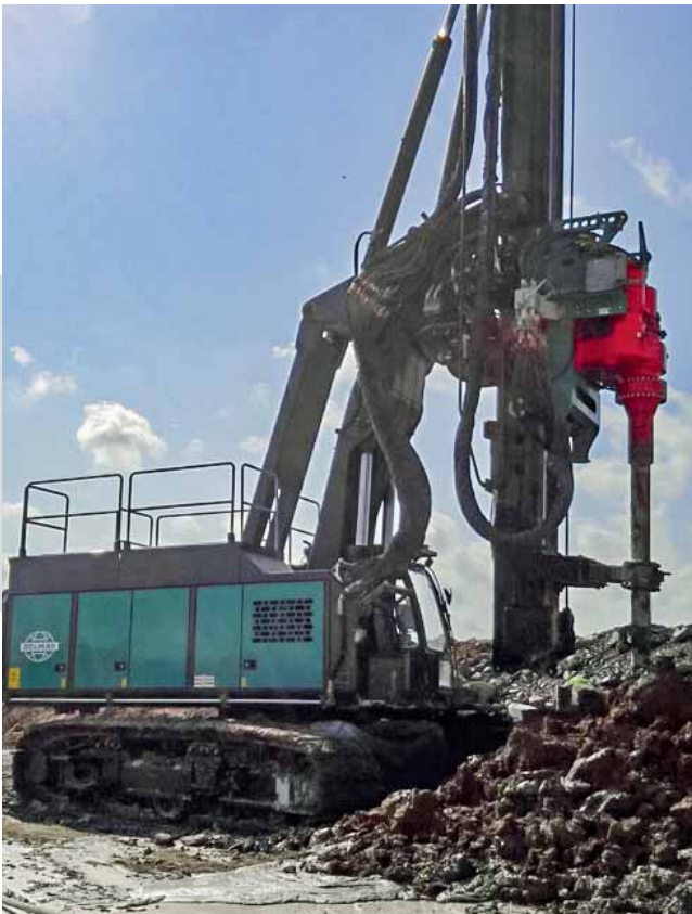
Soil mixing (WSM) using an RH 30 and RHP 150 auger drive to increase the load-bearing capacity of the soil. The existing soil material is mixed with a suspension additive.
