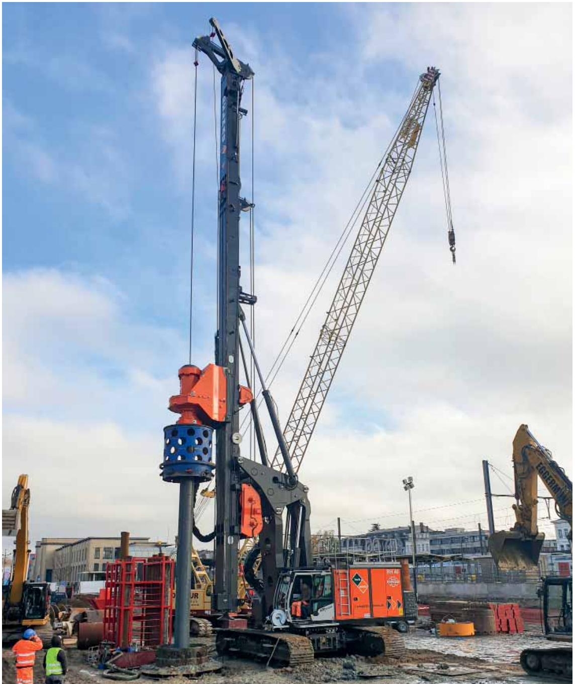
Drill rig RH 40 built on a T110 carrier for the production of drilled piles with a diameter of 1800 mm and to a depth of 40 m using the Kelly drilling method.
