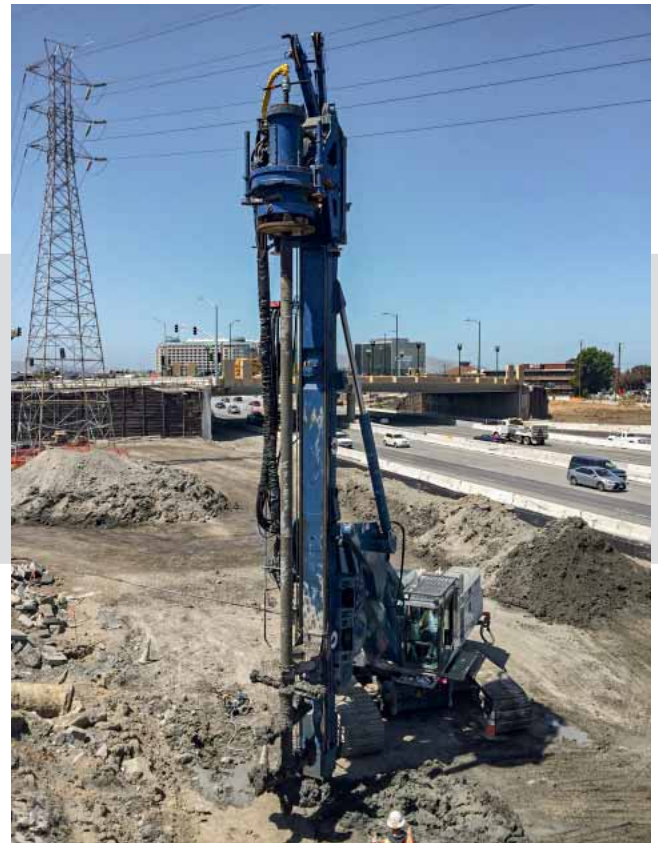
Drill rig RH 24/270 in a short leader mast application with limited headroom: The required depth is achieved by installing additional pipe sections on the mixing rod.
