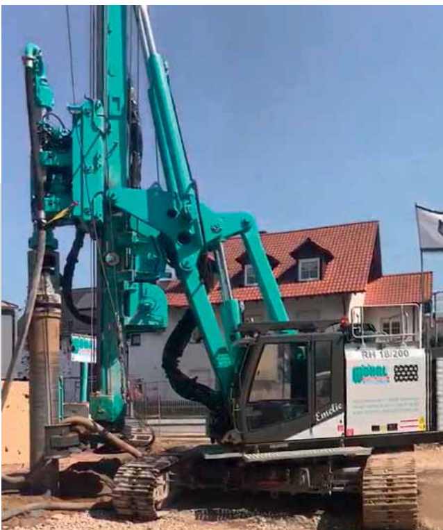
RH 18/200 during VDW drilling: The pile is created in a single pass. Immediately after reaching depth the concreting takes place and continues during the extraction process.
