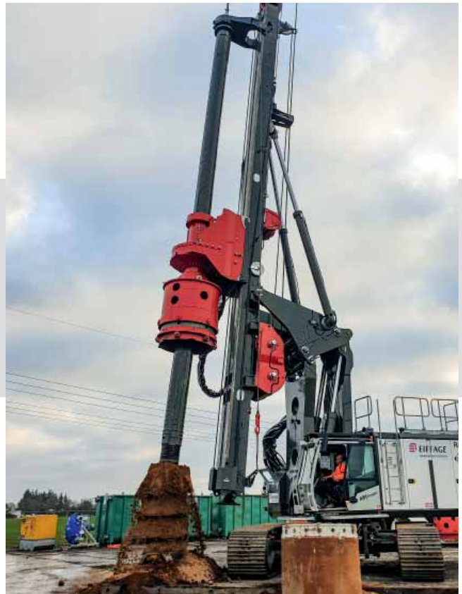
RH 40 with Kelly bar guide: In the case of inclined piles, the Kelly bar is also guided at the upper end to prevent the Kelly bar from tipping.
