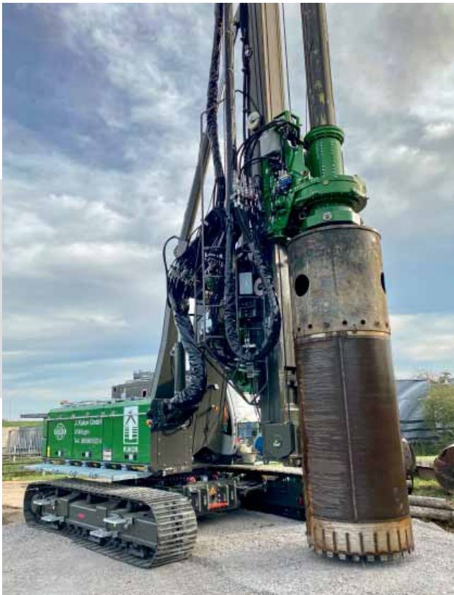
Drill rig RH 24/270: The telescopic undercarriage is equipped with mechanical connections for a casing oscillator (with an integrated control unit) for assisting in inserting large diameter casings in difficult soil conditions.
