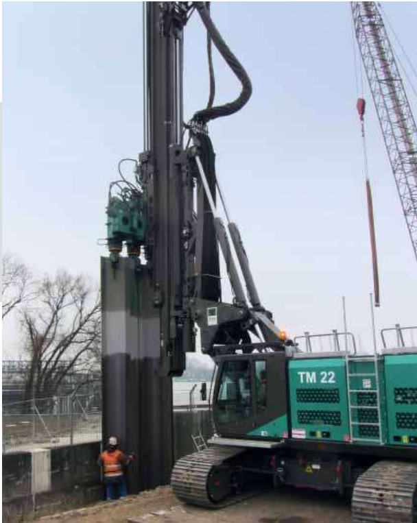
Using the Hydro-Press-System HPZ four steel sheet piles are pressed in a step sequence into the ground.
