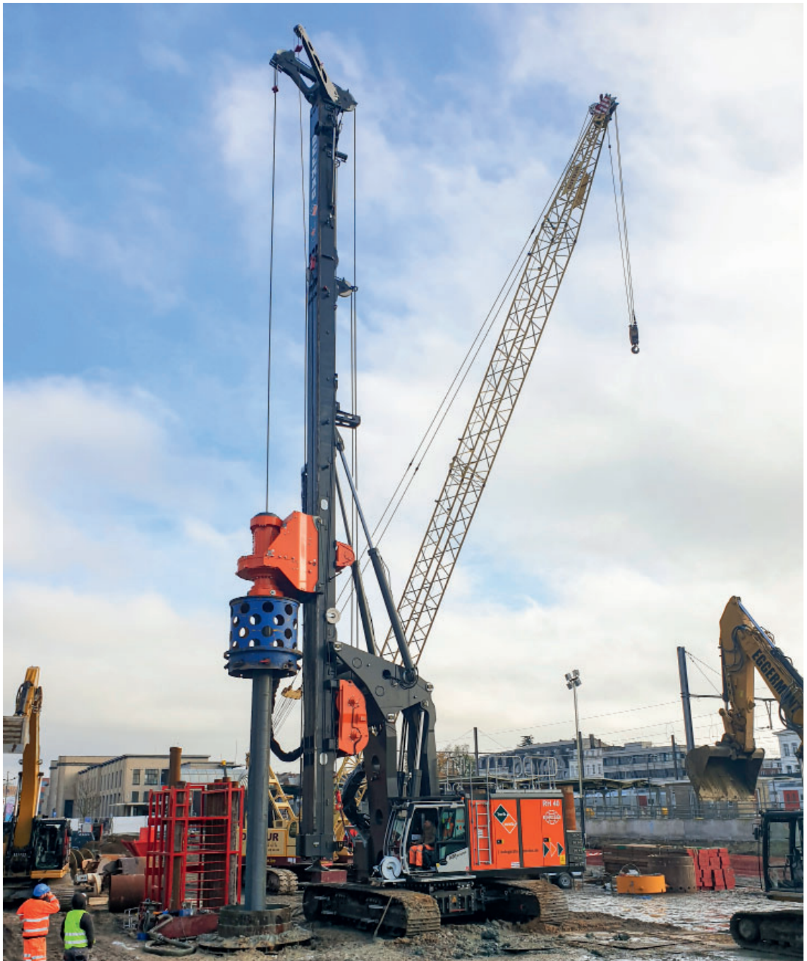
The biggest model of the DELMAG rotary drill rigs built on an ABI T110 carrier for the production of drilled piles with a diameter of 1800 mm and to a depth of 40 m using the Kelly drilling method.
