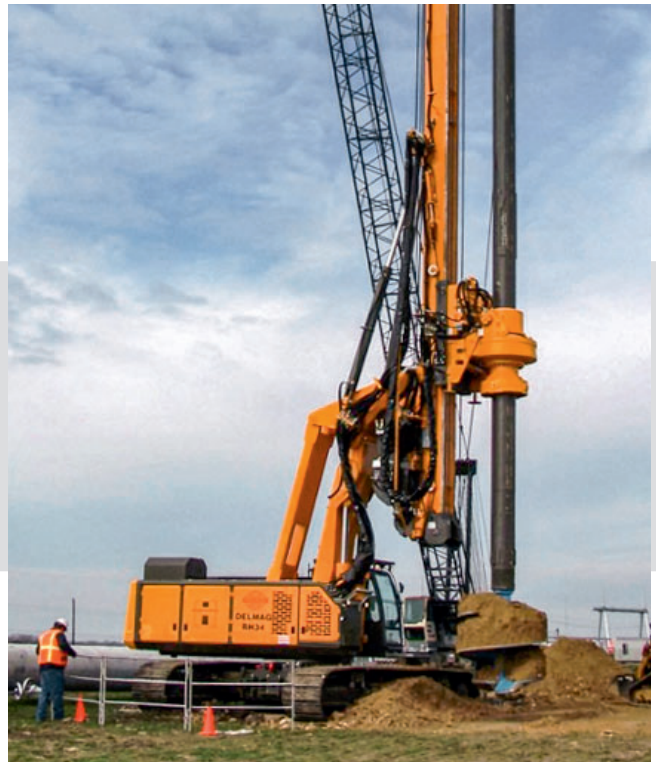
Uncased Kelly drilling with a short leader mast foot: The short leader mast foot enables larger diameters to be drilled, as the drilling tool can rotate underneath the leader mast.
