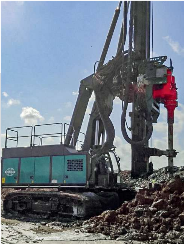
Soil mixing (WSM) using an RHP 150 auger drive to increase the load-bearing capacity of the soil. The existing soil material is mixed with a suspension additive.
