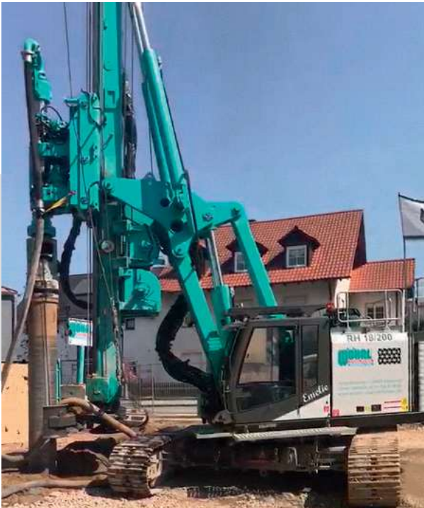
DELMAG drill rig during VDW drilling: The pile is created in a single pass. Immediately after reaching depth the concreting takes place and continues during the extraction process.
